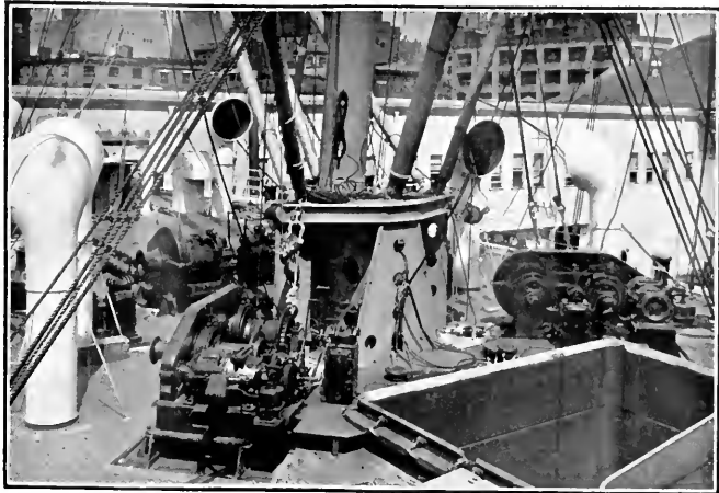
Electrified Cargo Winches of the new Ward Liner Morro Castle, equipped with Westinghouse 25 and 35-hp. Waterproof Motors and Waterproof Cam Type Control. Westinghouse Waterproof Motors for deck machinery are the most rugged type built—especially designed for hard usage in port and heavy weather at sea. They are noted for their reliability, quick starting and stopping, water-tightness, low maintenance and long service.
